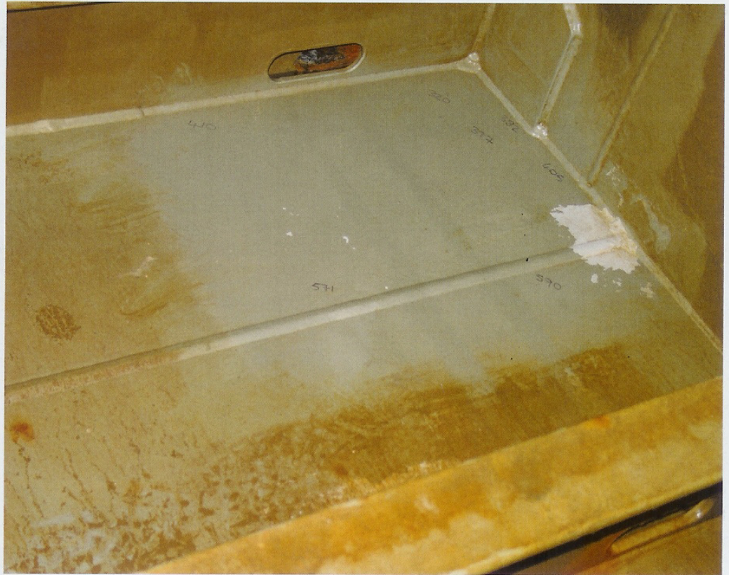
Intershield 300 in a ballast tank after 13 years of service.
